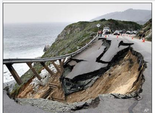
A section of the southbound lane of Highway 1 slides down the hillside on Wednesday, 16 March 2011 in Big Sur, California (© AP Photo/Monterey Herald, Orville Myers)
